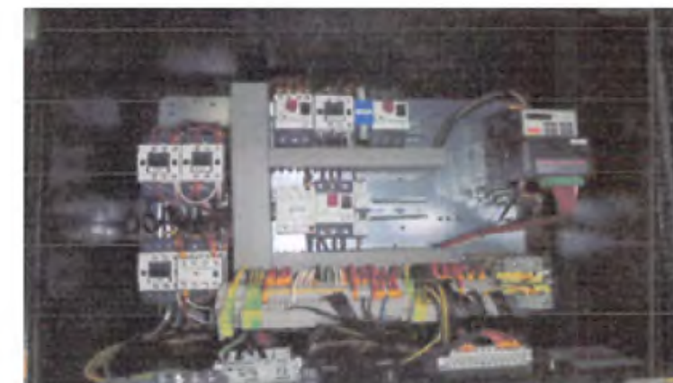
Panel Maintenance Service
